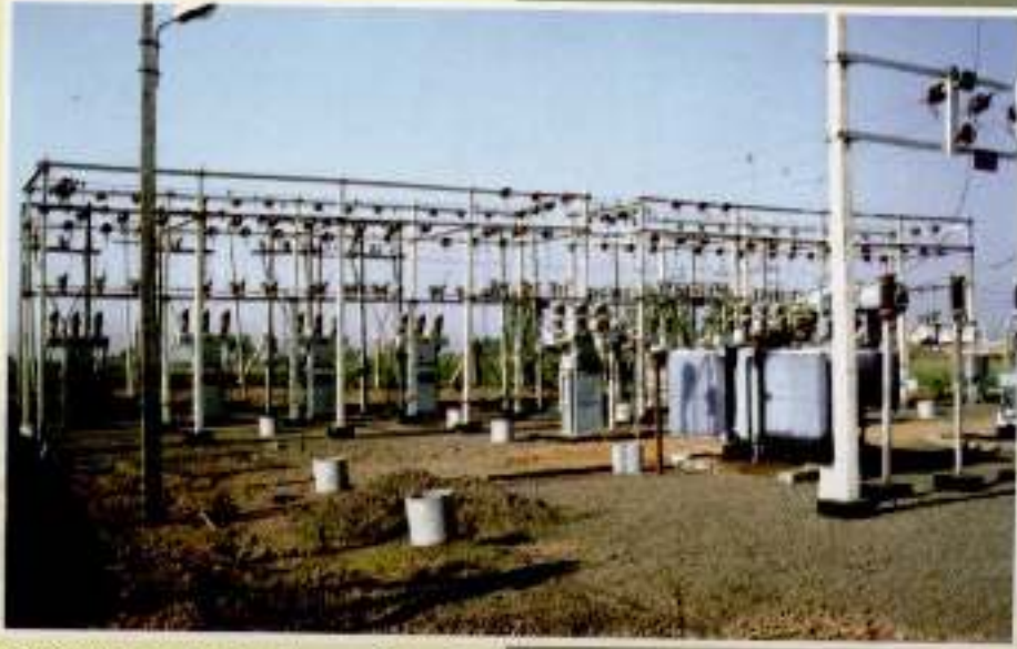
33KV Nanadi Sadalaga Sub-Division, HESCOM Division, Chikkodi.
